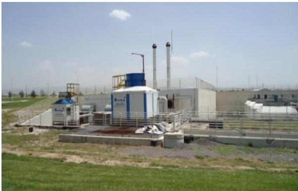
Figure 5. Esenboga Airport Tri-Generation Plant [2]
