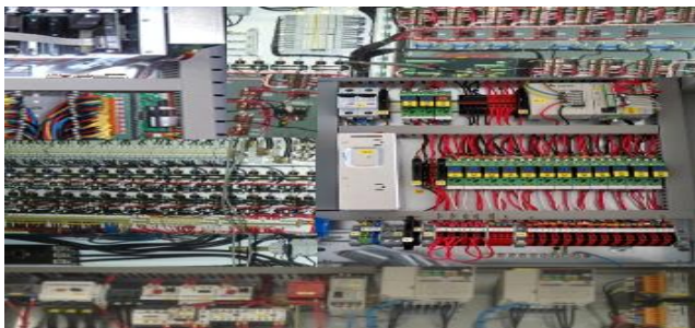
Figure 8. Established security panel
