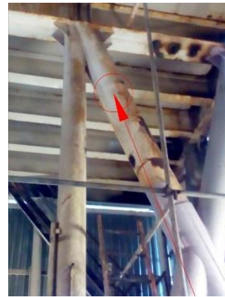
Figure 4. Damaged inclined distribution pipe
