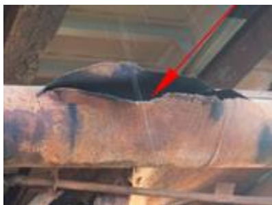
Figure 3. Damaged horizontal distribution pipe
