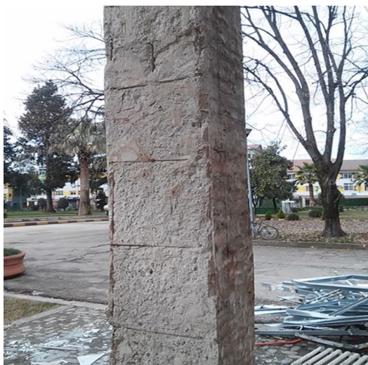
Figure 4. Column on the ground floor displaying visible indications of iron bar corrosion
